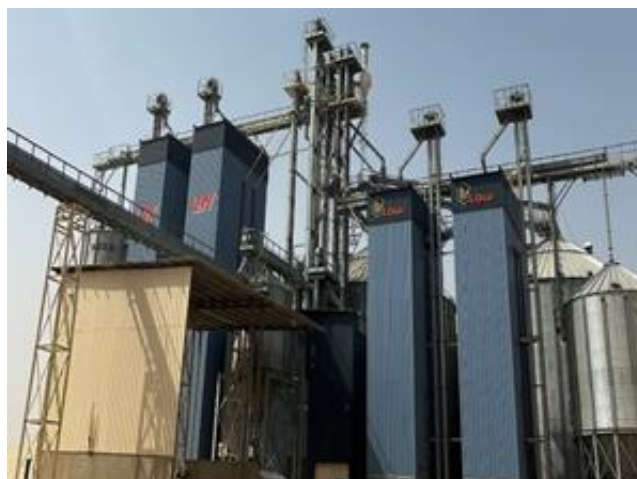
Exterior of a rice processing plant in Senegal. Photo Credit: Laura Courbois / MarketShare Associates
